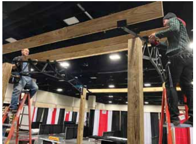
Steel trusses are also much more resistant to warping, fire, and heat damage than wood trusses.
