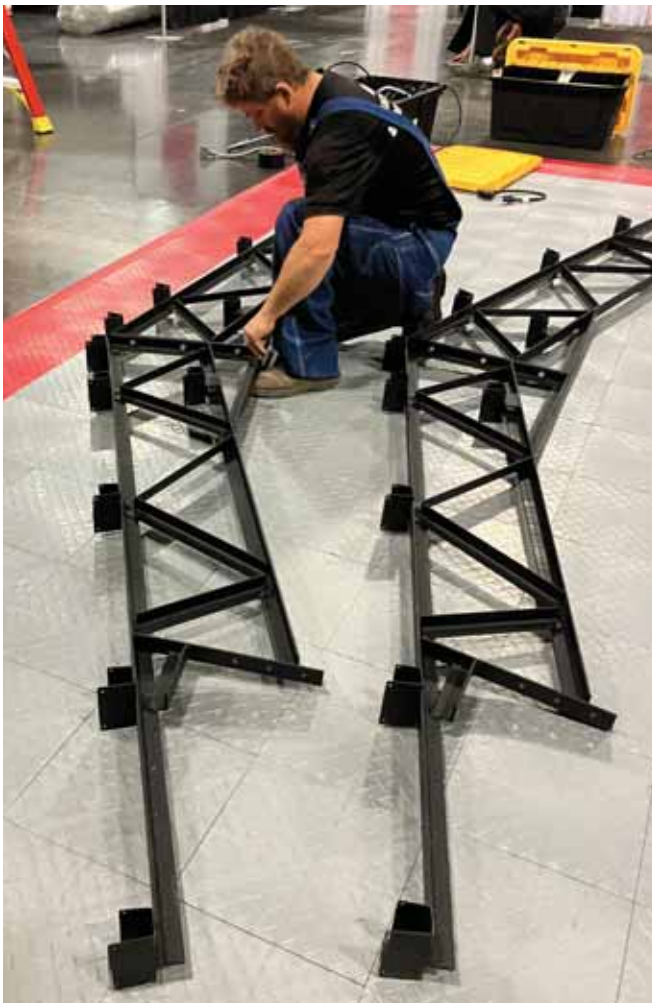
Steel trusses require fewer posts, trusses, and concrete, which reduces material and labor costs.
