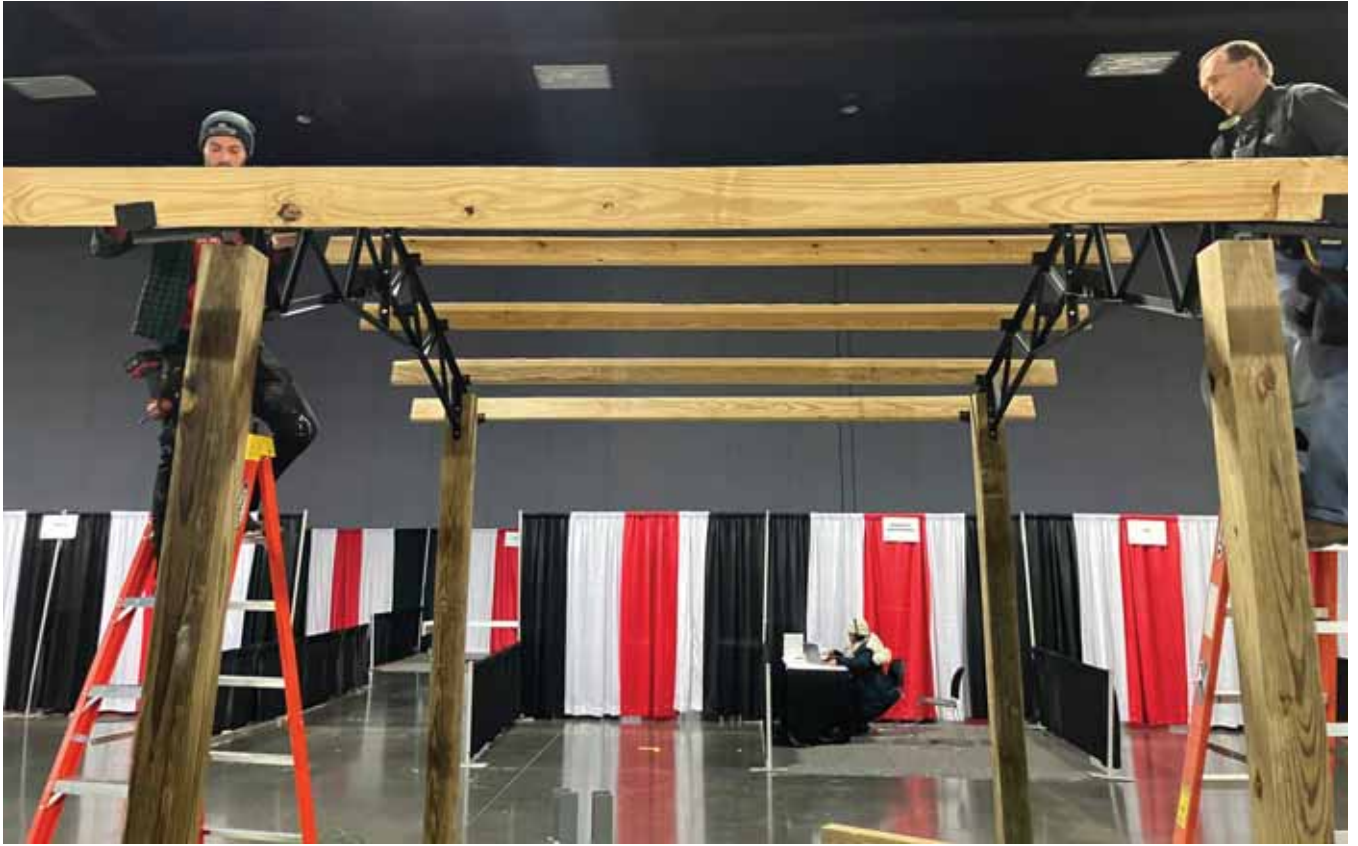
Steel trusses can span a much further distance than wood trusses, allowing for more usable, support-free space.
