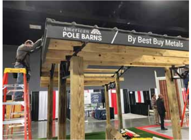
The Best Buy Metals booth nears completion after just a few hours. Steel trusses made this project practical for a temporary structure.
