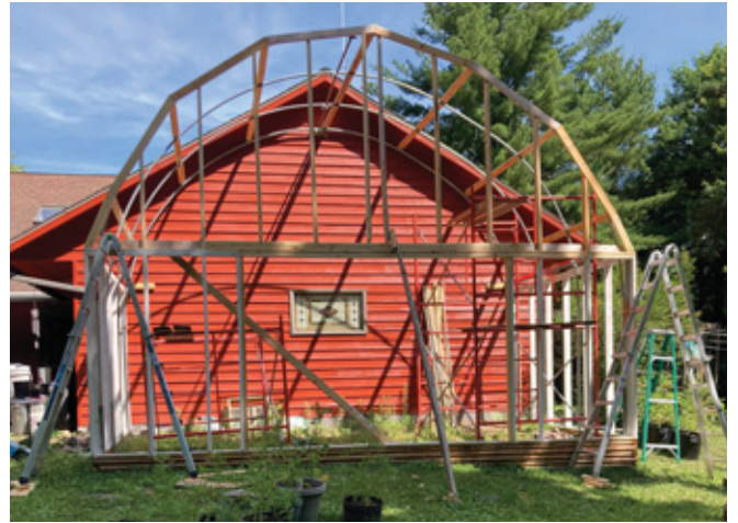
The author wound up with two studs over the center door (oops).
