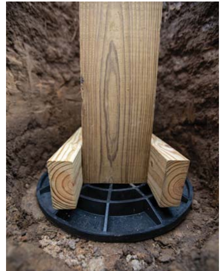
FootingPad is always placed flat side down into the hole. Shown here, uplift brackets are attached to the post. PHOTO COURTESY FOOTINGPAD, WWW.FOOTINGPAD.COM
