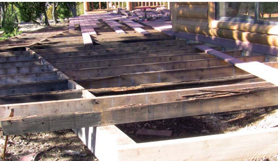
Here, you can see how the joists were rotting away beneath the composite decking, which had no indication the deck was rotting away.
