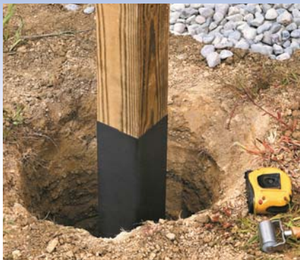
Protecting the post from 2" above grade to 6" below grade will eliminate below-grade decomposition of the wood.
